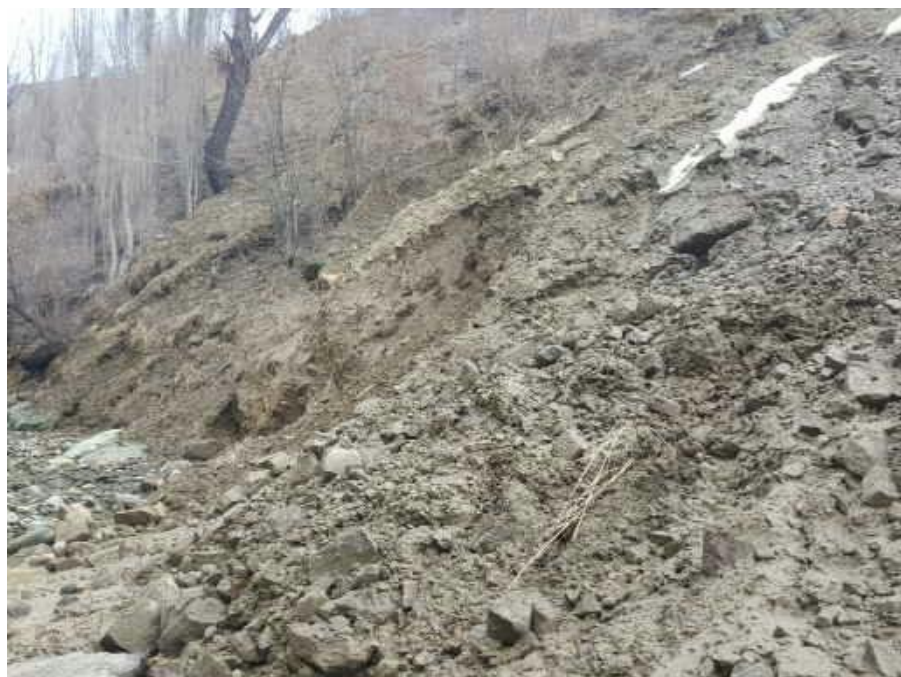
Figure 1 Weathered, shattered and jointed loose strata with high slope
