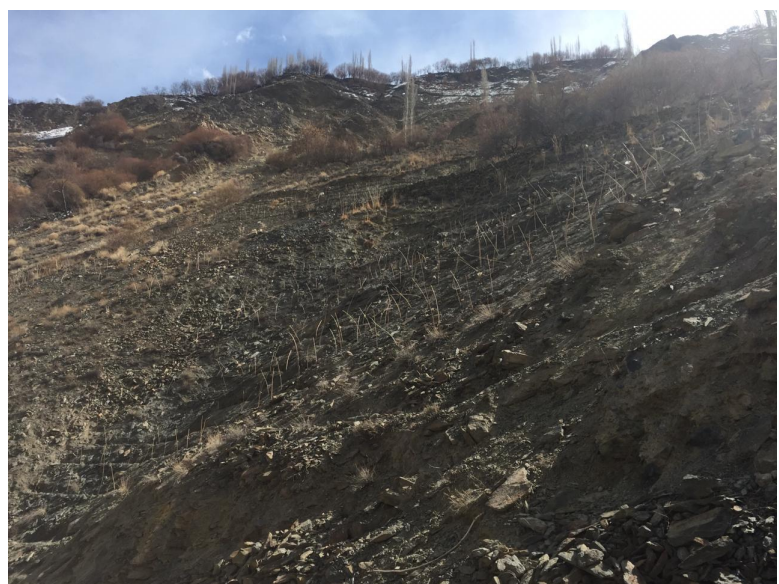
Figure 3: Weathered, shattered and jointed loose strata with high slope
